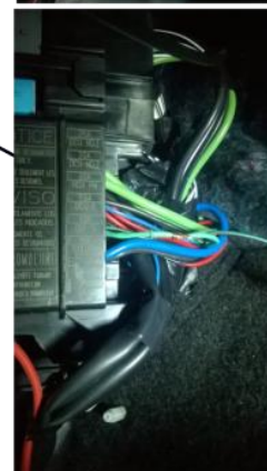
Window heater signal
